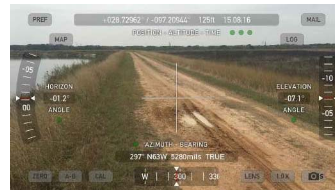
2306 - Top of Levee - Minor Ruts
