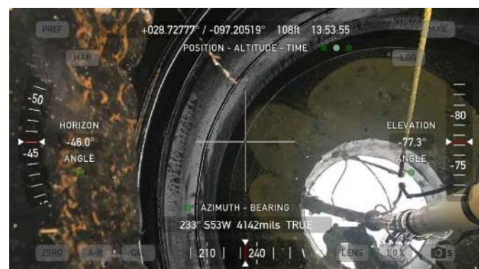
2180 - Silted Inlet to Sump
