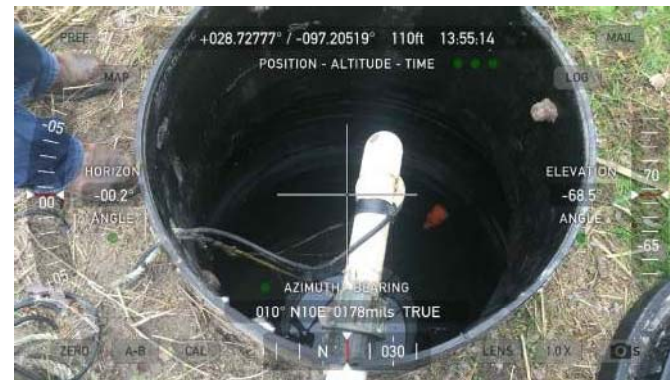
2186 - Seepage Collection System Sump
