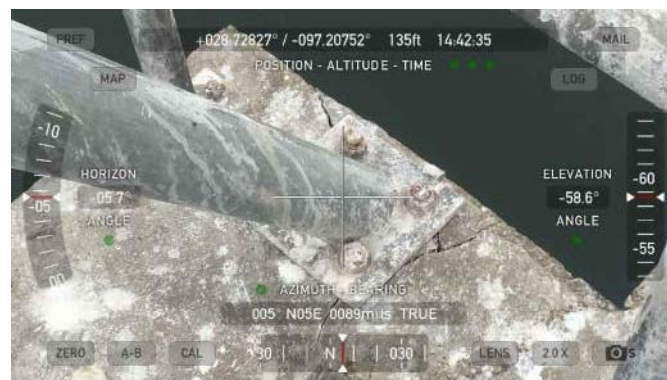
2243 - Rusted Handrail Bolts and Cracked Concrete - Handrail is Loose
