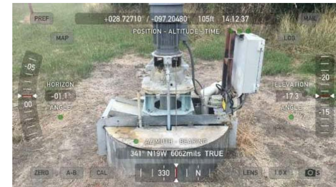
2199 - Seepage Collection System Sump
